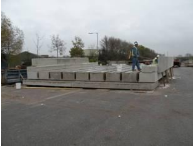
Above: Looking towards Broadway from the track bed and the deck of the new bridge
